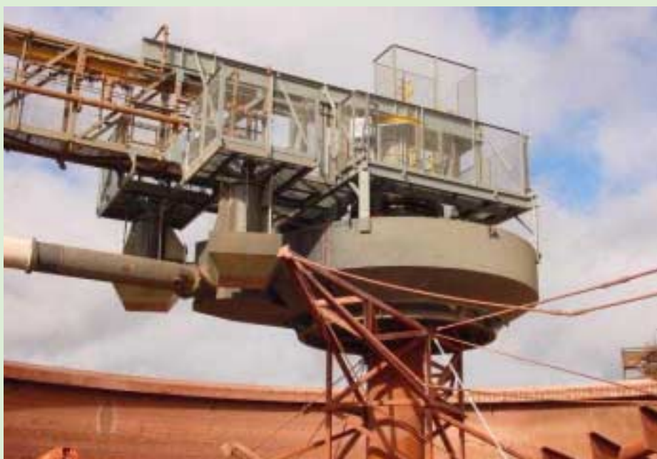
Rake lift system and feedwell of an existing laterite counter-current decantation system.
