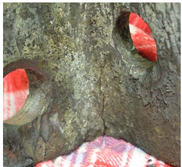
Figure B4 – Crack in cleat (S2-SG27-dn-south)
