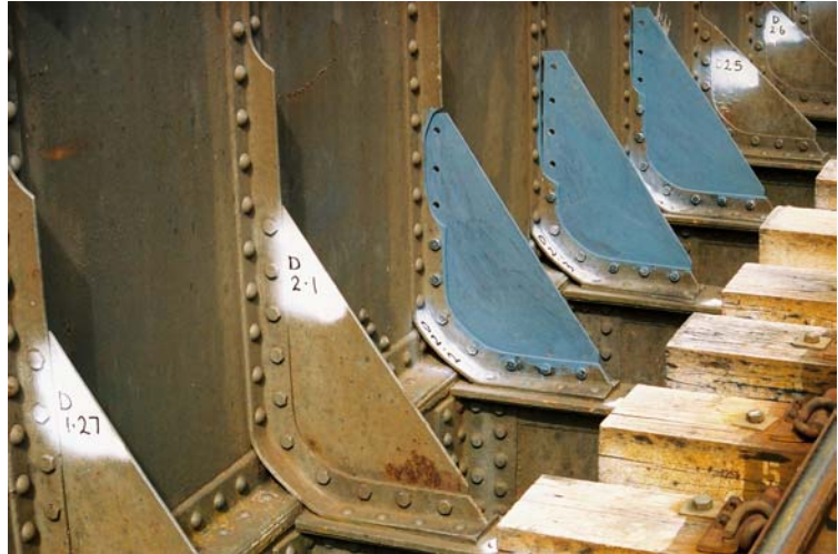
Figure B6 – Secondary cross girder connection to box girder, with original and replaced gussets
