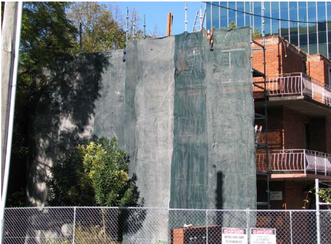
Demolition work being carried out recently to make way for a competition winning office building in the Parramatta CBD
