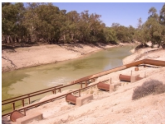
Figure 2: Pipe discharge to the Darling River
